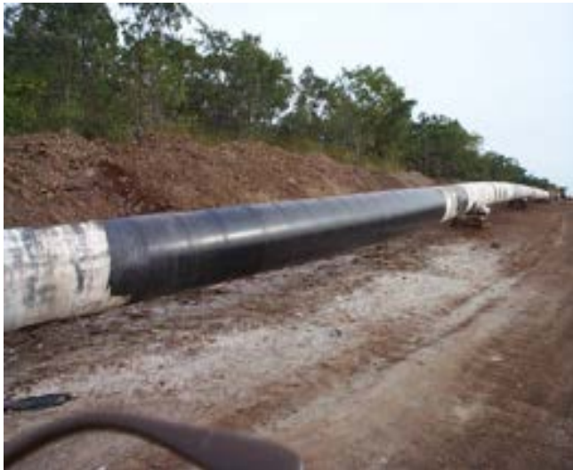
CONTINUOUS HEAT-SHRINK SLEEVES APPLIED OVER A SECTION OF DAMAGED ASPHALT PIPELINE COATING
